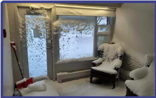
Photos of RMC Kingston Broken windows in the Tailors building
